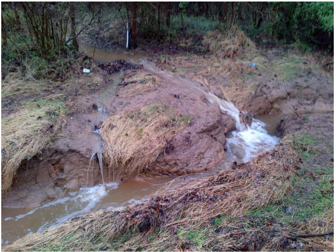
Existing conditions showing unstable stream at Sawmill Creek
