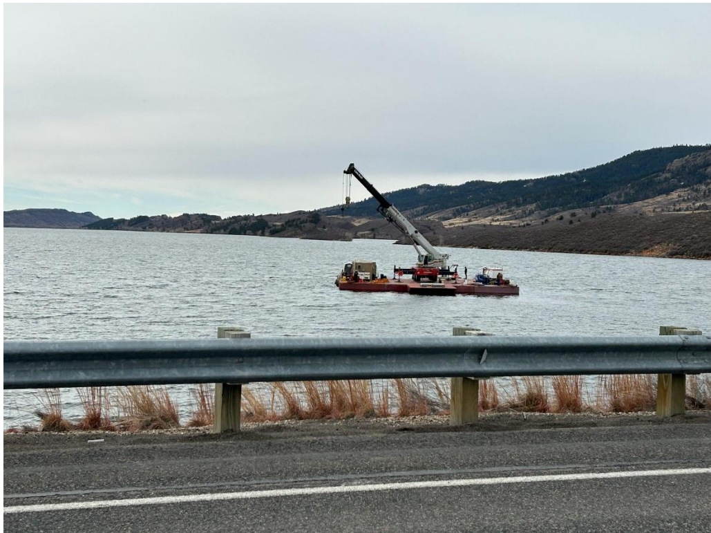
Above, a barge equipped with a crane that could lift the heavy bulkheads was used on Horsetooth Reservoir in March for the bulkhead testing.
