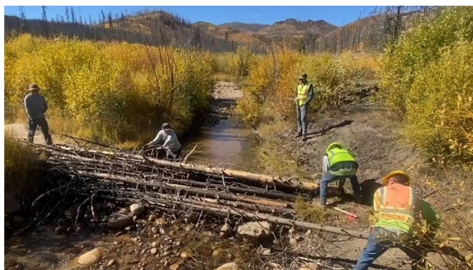
Crews placed post-assisted log structures (PALS) on Forest Service land within the burn area of the 2020 East Troublesome Fire.
