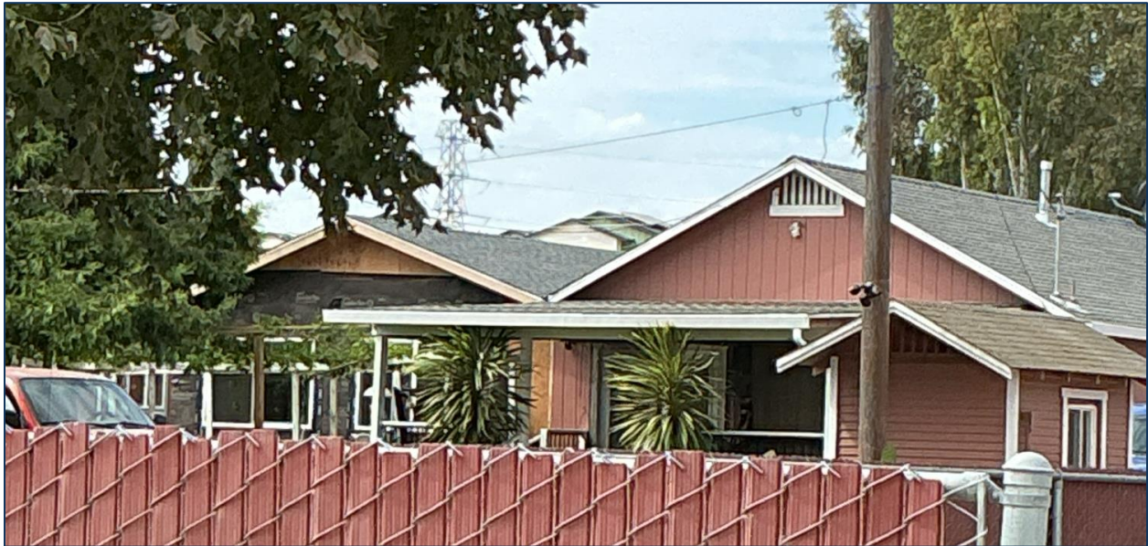
Figure 2 – Picture of Home and Addition with Visible Exposed Plywood
