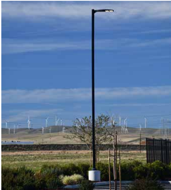
Typical Single-Head Parking Lot Lighting
