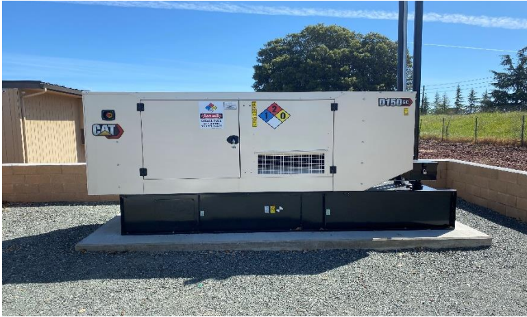
E. Recreation Center Emergency Generator Project
