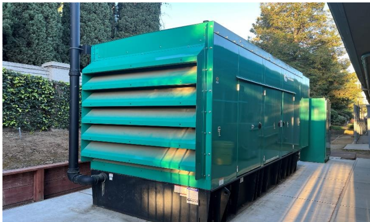
D. Civic Center Emergency Generator Project
