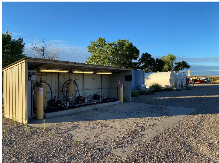
Figure 1: Existing fueling infrastructure.
