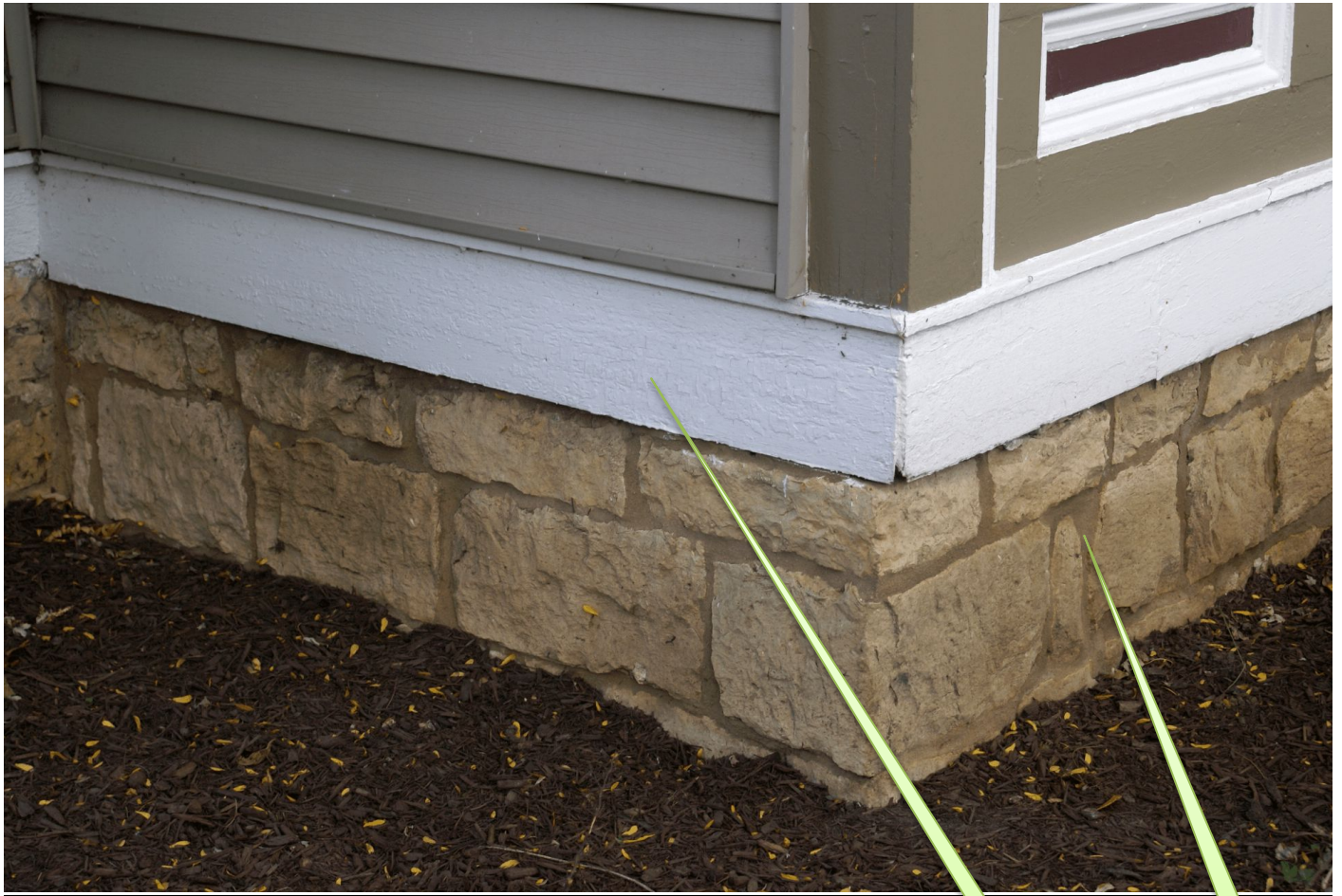
Plate 14 – Bottom corner typical condition photo credit: Leif Hendricksen
