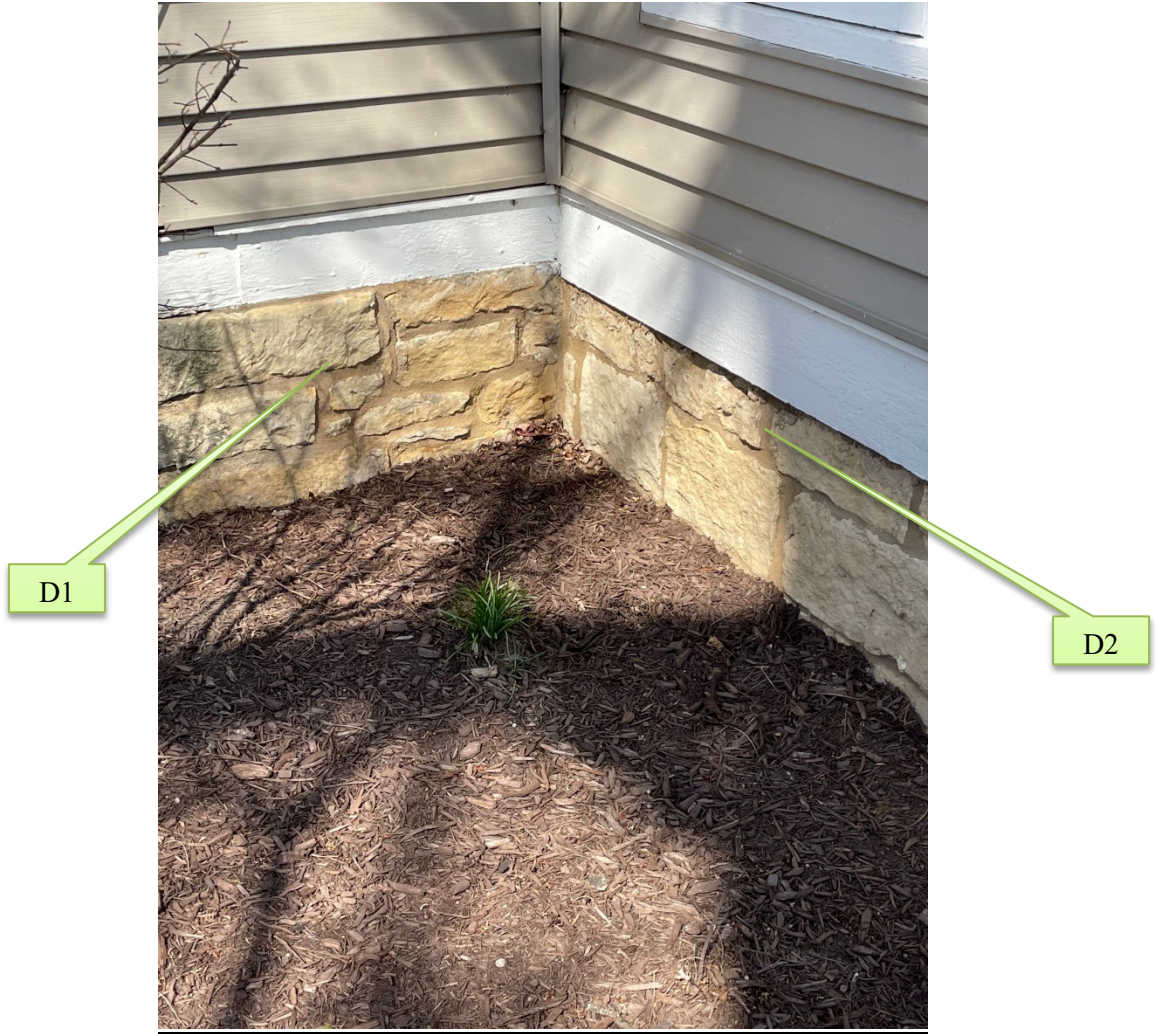
Plate 16 – Foundation detail (connection at original upright and 1-story bay addition) photo credit: David Schmidt
