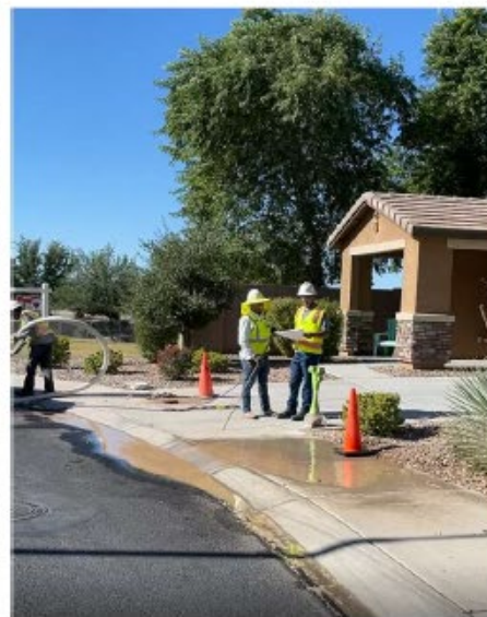
Pothole and Clean up
