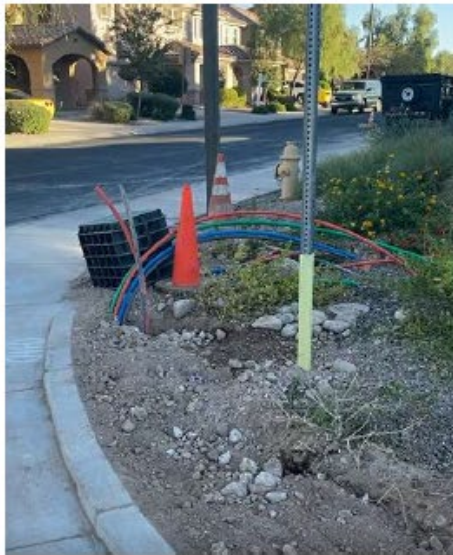
Handhole at the edge of neighborhood
