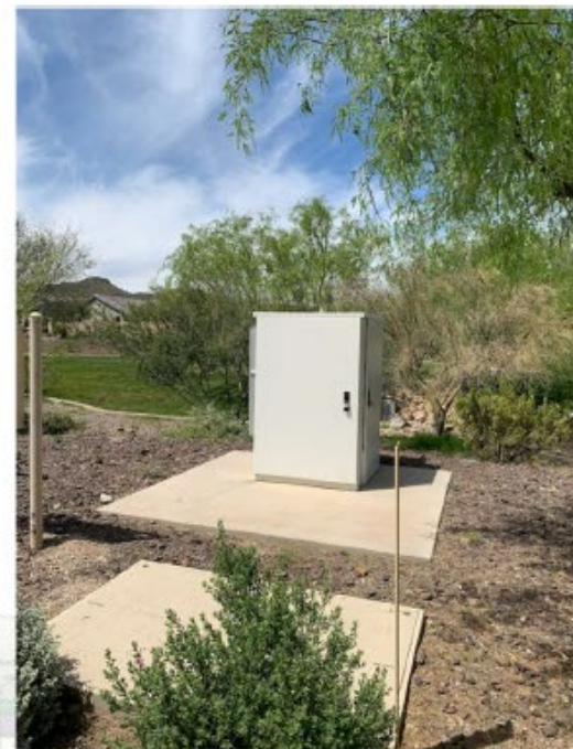
One Cabinet to Serve 10k+ homes
