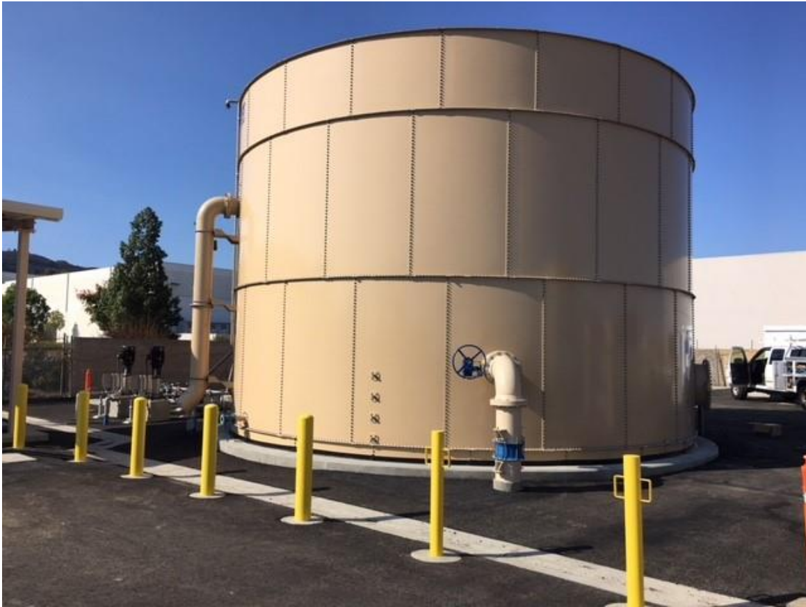
Backwash Tank for Existing Iron-Manganese Treatment System at Well No. 102
