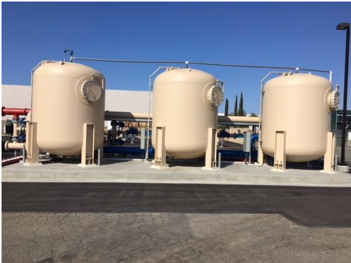
Pressure Vessels for Existing Iron-Manganese Treatment System at Well No. 102
