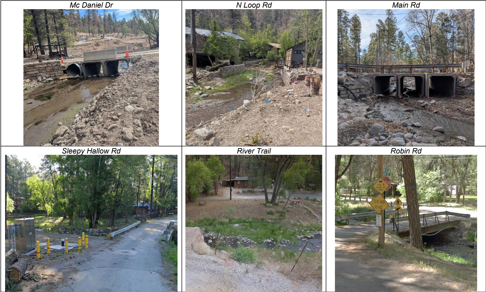
Figure 1 - Existing Bridges Condition
