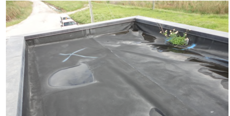
S-250S: Blisters and moisture under roof membrane and vegetation growth in scupper
