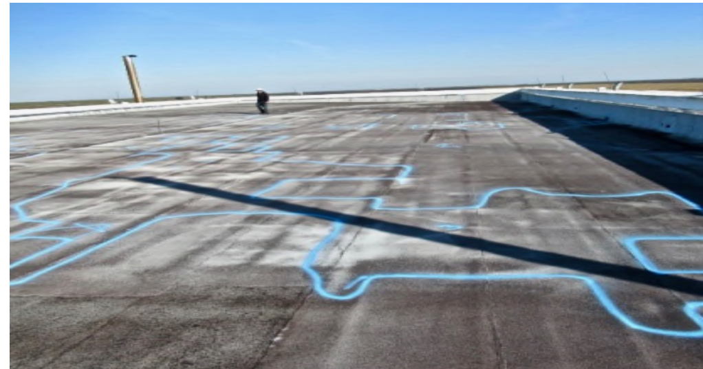
G-372: 16 large areas of wet insulation
