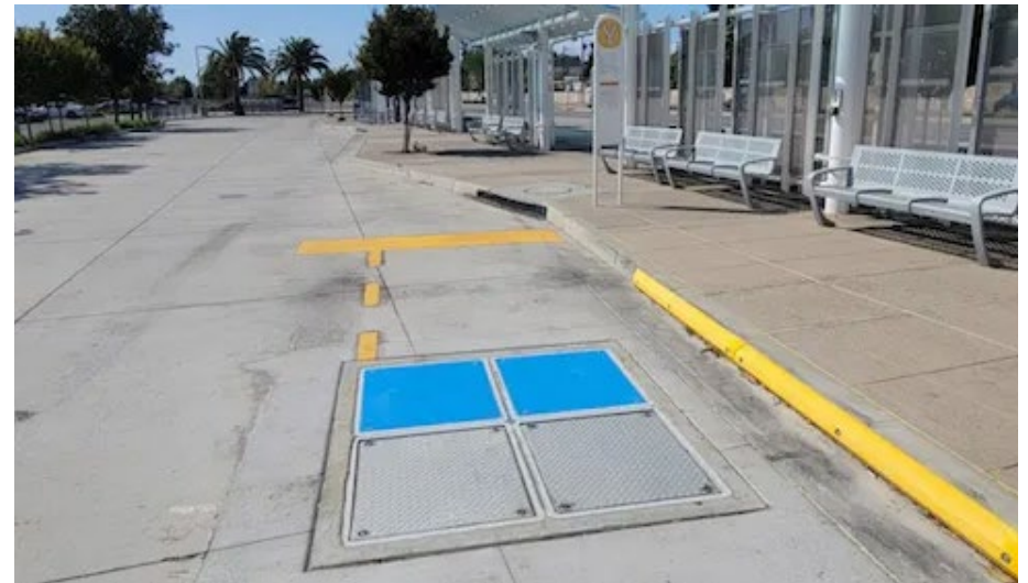
Figure 4-2. Inductive Charging Plate at Curtola Park and Ride
