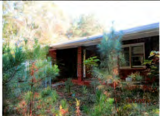
10.21.2014 - FIELD INSPECTION BY HARRY BUSBY FOUND IMP IN POOR CONDITION, INTERIOR DAMAGE, NO UTILITIES, HOUSE ABANDONED FOR PAST FIVE YEARS. SEE PHOTO FILE ON V DRIVE. L.L.
