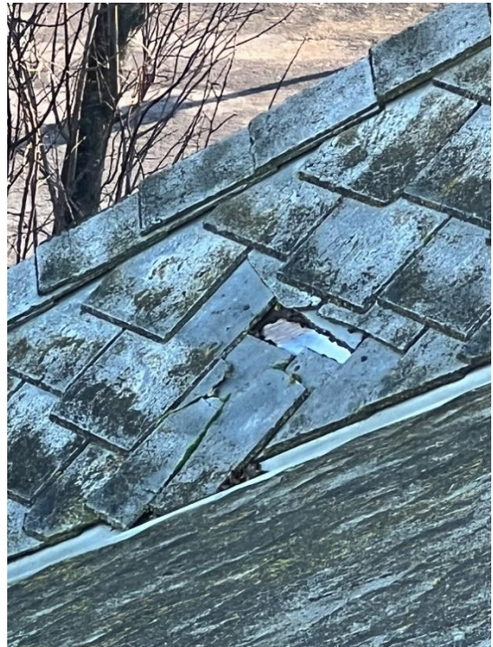
Broken Roof Tiles
