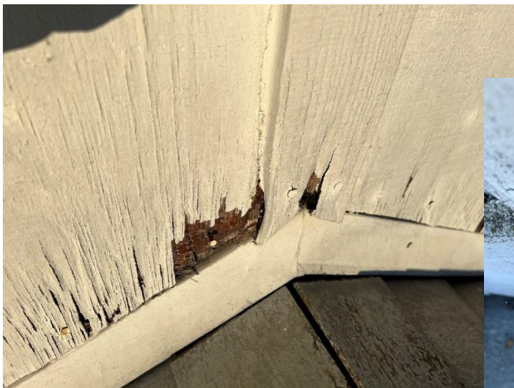
Parapet Wall Damage: Severe Dry Rot
