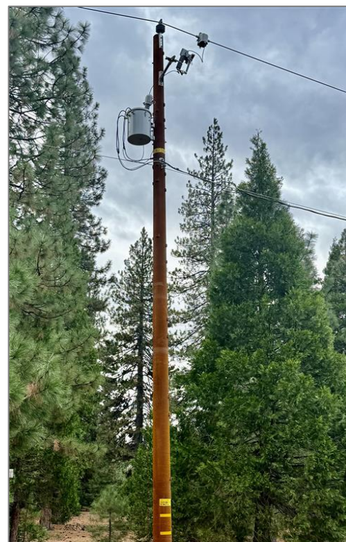
Figure 6-2: Distribution Steel Pole
