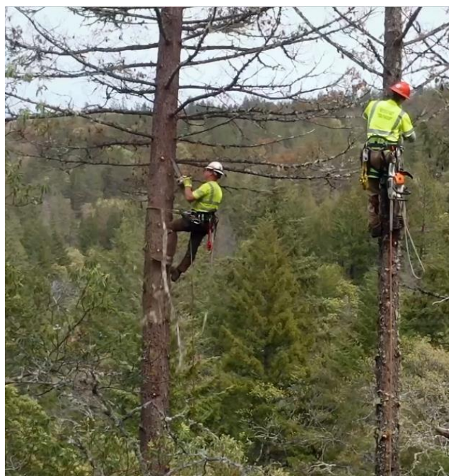
Figure 5-1: Hazard Tree Removal
