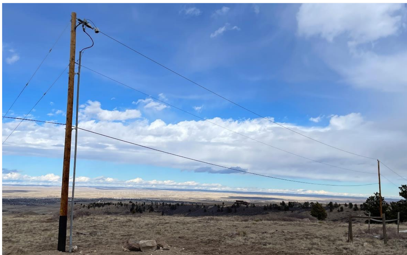
Figure 6-5: Lines Out of Community Park Substation Scheduled for Undergrounding
