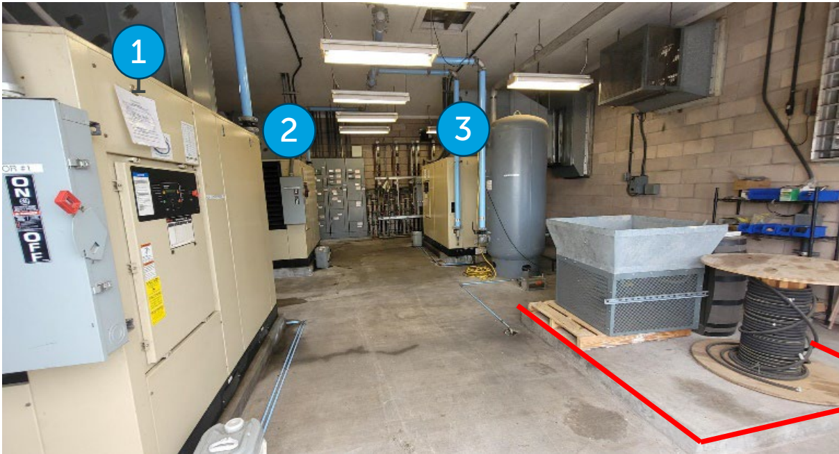
The three existing compressors to be replaced
