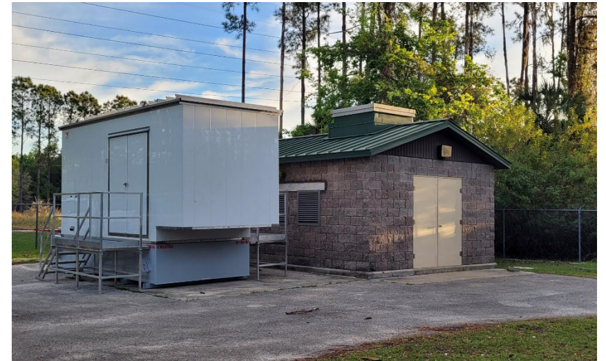
New generator at well 5
