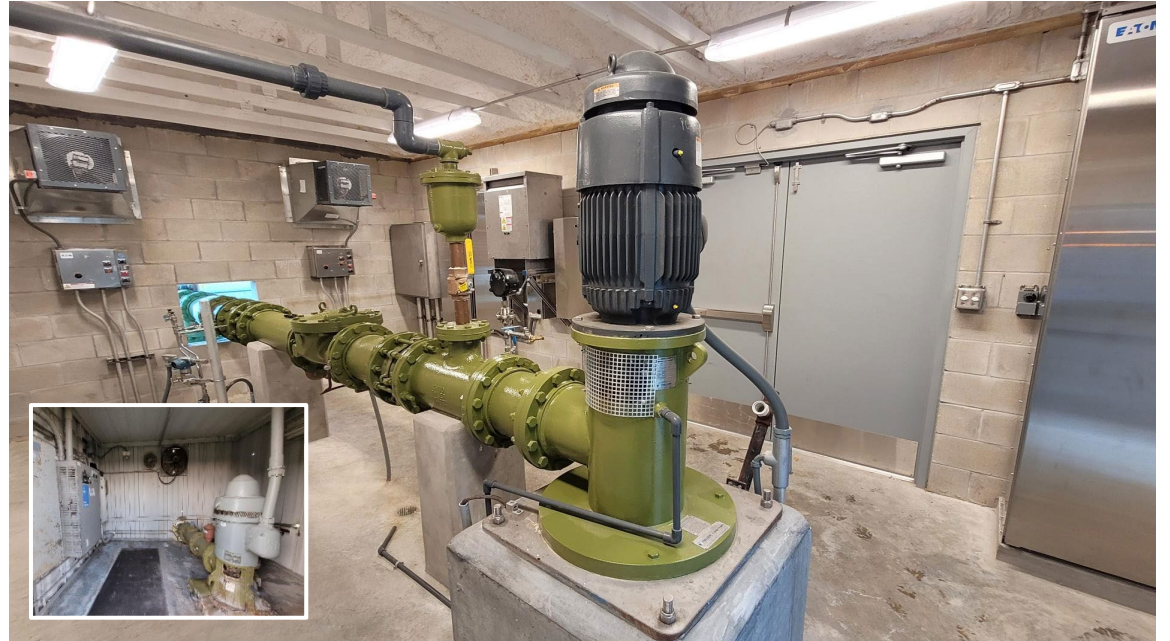
New pump and electrical equipment
