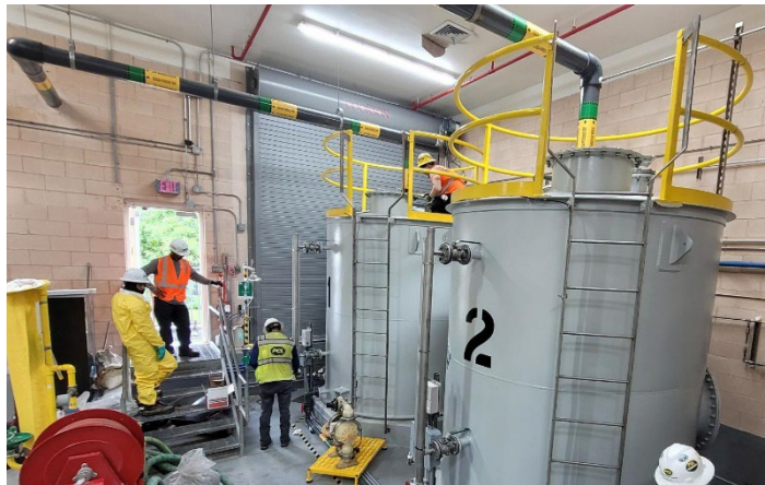
South Pasco Caustic Feed System
