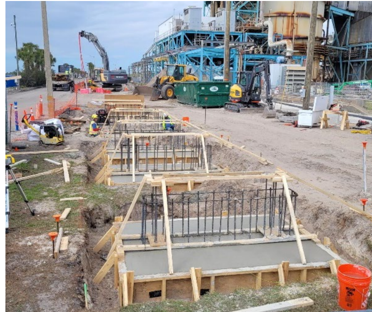
Concrete pipe supports for above ground 54" pipeline
