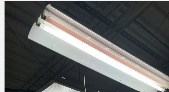
Public Works Burnt out T8
