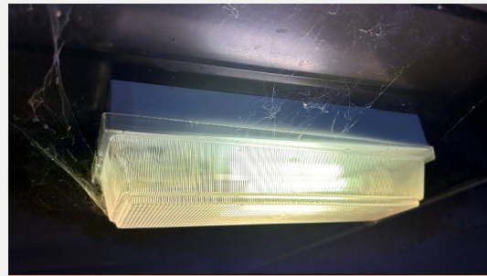
Fire Station #3 T8 Bulbs
