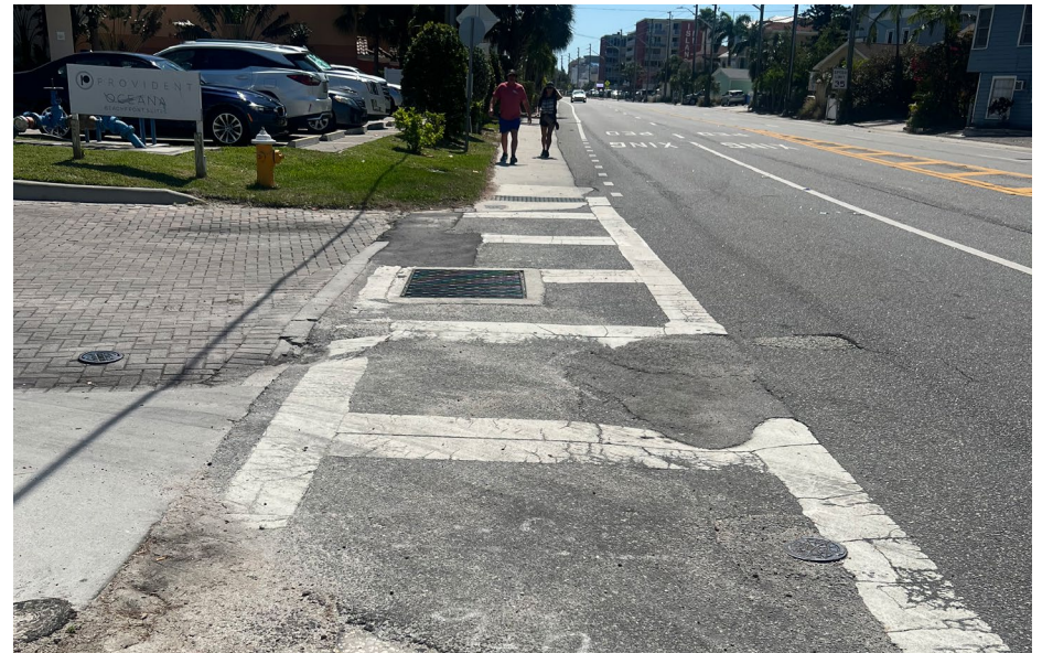
South Segment - Pavement Conditions: Faded crosswalks, drains within the pedestrian and bike paths, and pavement patches were common observations within this segment.
