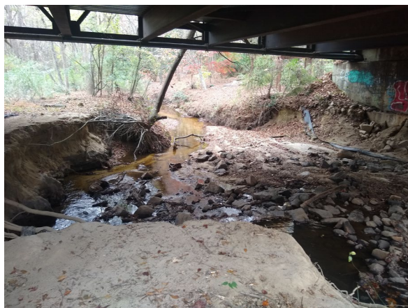
Figure 11. Severe Erosion on Toms Creek
