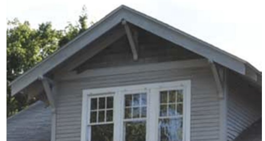
FIGURE 22: AS SEEN HERE, WINDOWS ARE INTEGRAL TO THE HISTORIC STYLISTIC CHARACTER OF HOMES. THE CHARLES AND GERTRUDE RAWLS HOUSE, AT 545 HAYES STREET, HAS WINDOWS THAT UTILIZE MUNTIN DESIGN TYPICAL OF CRAFTSMAN BUNGALOW—THREE DIVIDED LIGHTS OVER ONE.
