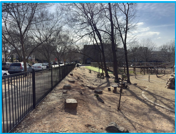
View: Eroded Slope Along Market Street
