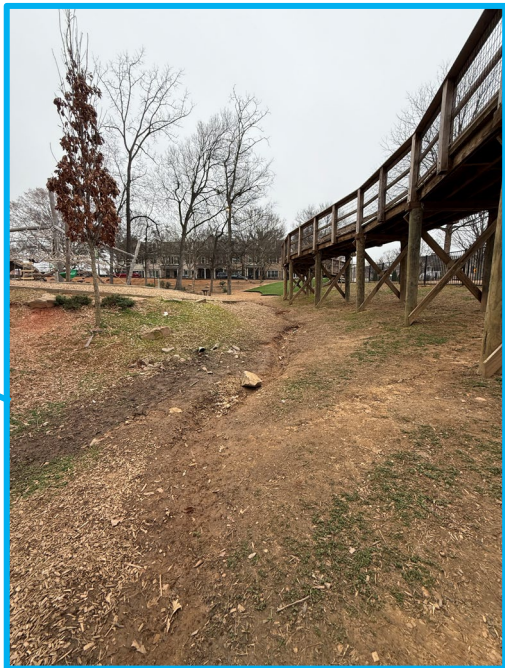
View: Eroded Swale Along Maple Street
