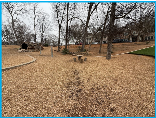
View: Eroded Swale at Toe of Slope
