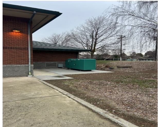
New emergency generator at Station 93
